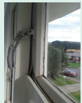
Figure 2. Missing window fittings.
