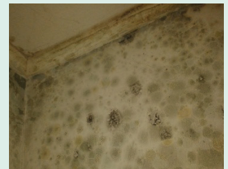
Figure 1. Extensive harmful mould in the wardrobe in the unused bedroom.
